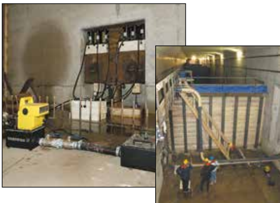
◀ The unique Enerpac RA-Series cylinders – lightweight and made of aluminium alloy – these RAC506 cylinders are ideal for the positioning of tunnel elements under the river (High Speed Train Line, The Netherlands).
