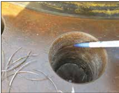
▲ A typical thread before refurbishment
